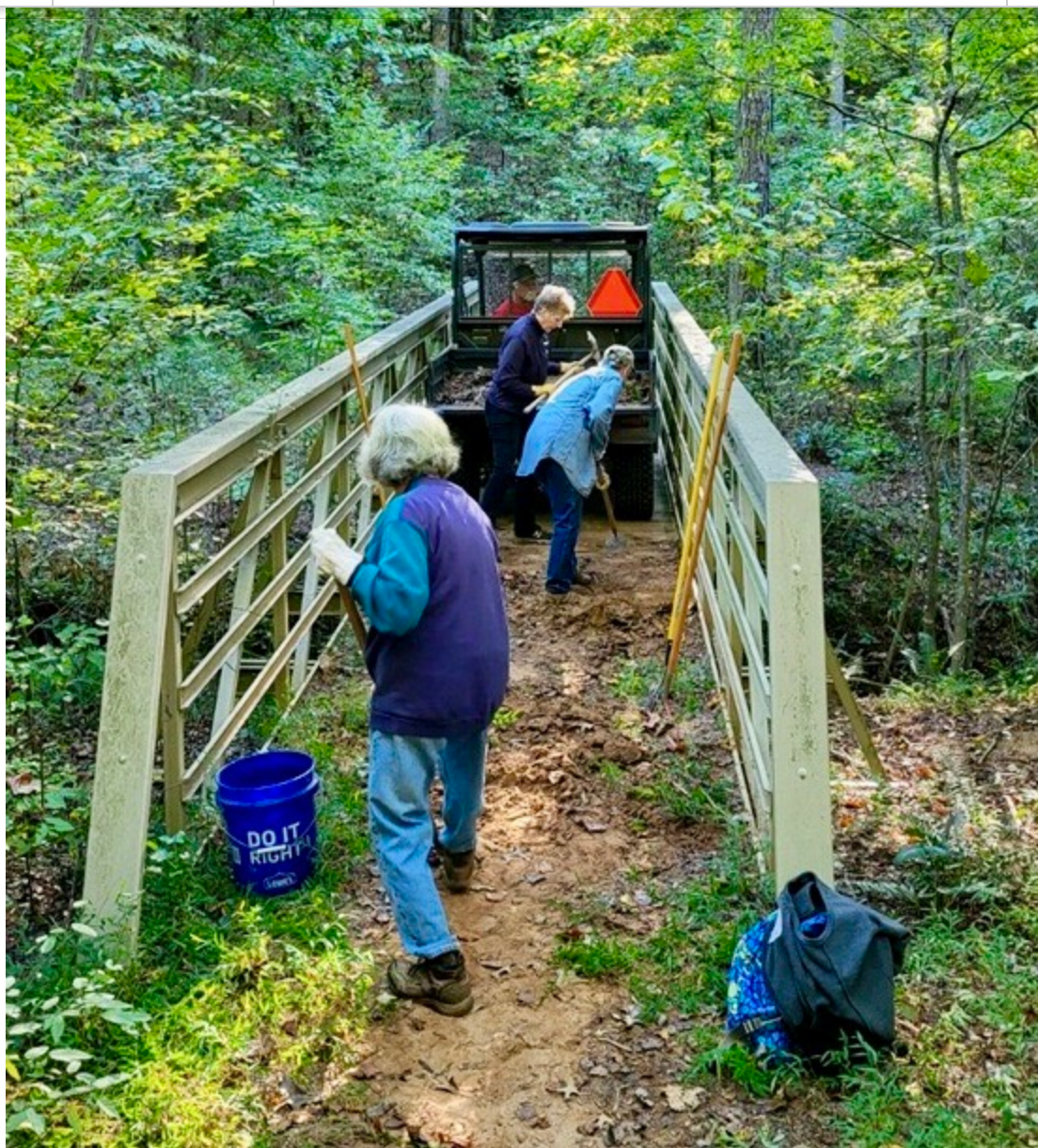
During the September 24 Heritage Park Work Day, bridge 3 was cleaned to remove thick accumulations of dirt and plant roots from the wooden boards. This work will help prevent the wood from rotting. Jeanne, Lori, and Lisa are shoveling, and Wendell is manning the Kubota.
